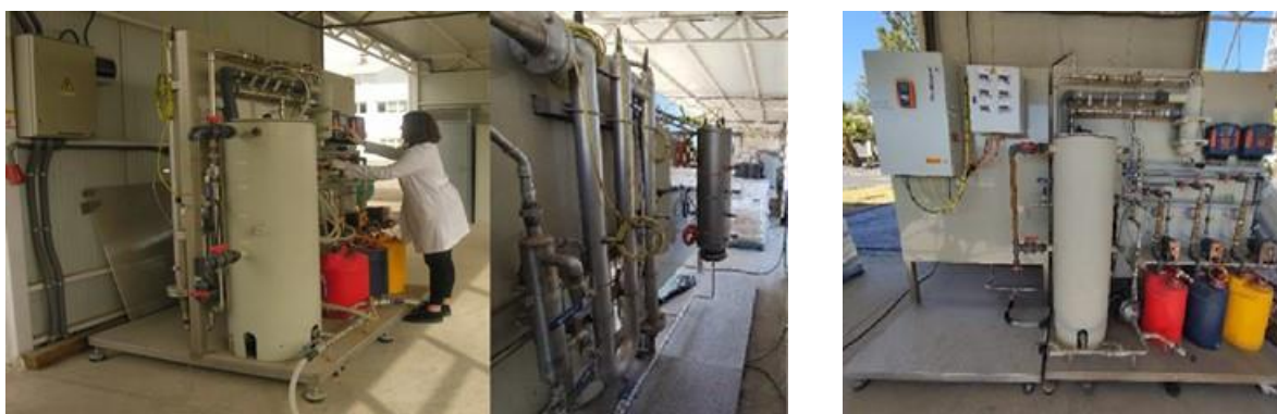
Figure 96. (Left) UVC pilot plant installed at PSA facilities and (Right) recent improvements.
