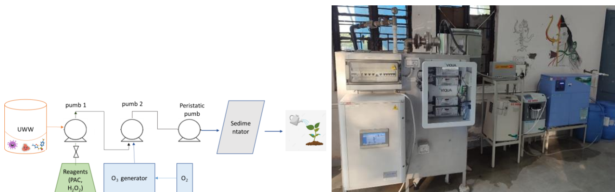
Figure 37. (Left) Diagram and (Right) picture of the Multifunctional Reactor (MFR) installed at MES GE Air Force Sewage Treatment Plant (STP).
