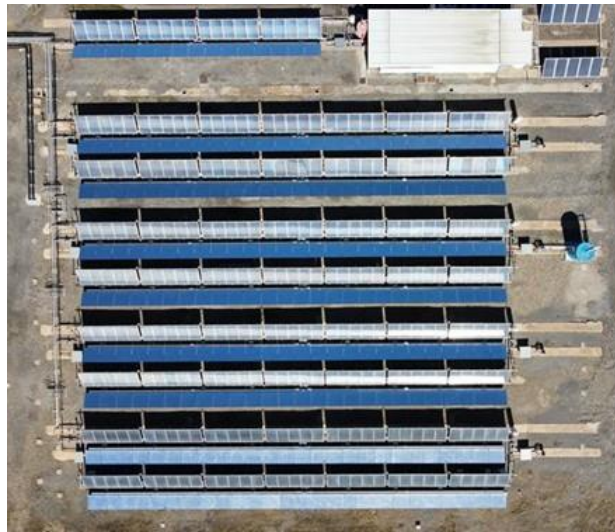
Figure 83. Aerial view of the 606-m 2 large-aperture flat plate solar collector field (AQUASOL-II).
