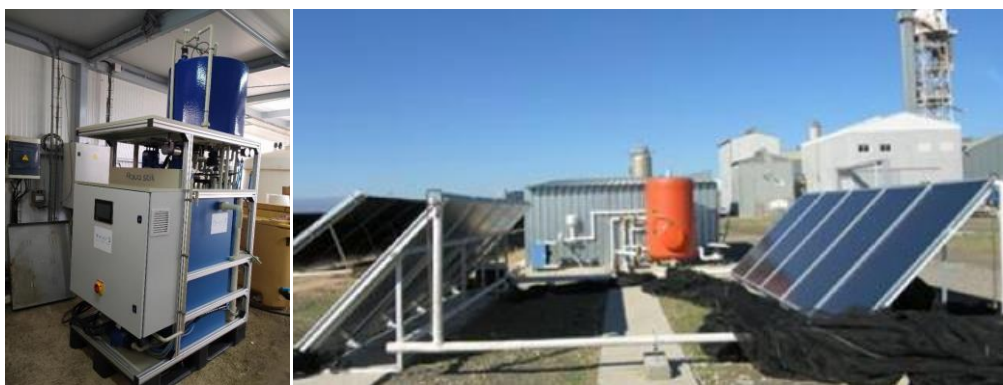
Figure 85. Internal (Left) and external (Right) views of the Membrane Distillation experimental test bed within the PSA low-temperature solar thermal desalination facility.
