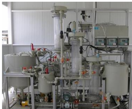
Figure 106. Biological pilot plant installed at PSA facilities.
