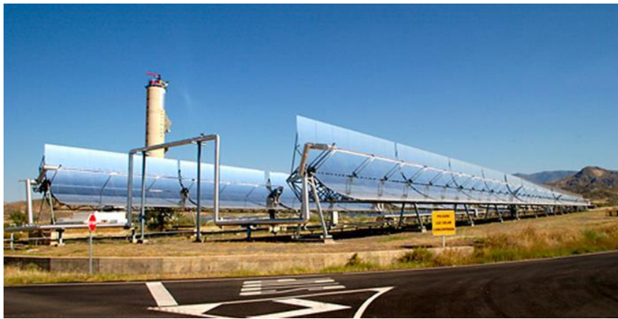
Figure 52. View of the DISS plant solar field in operation.
