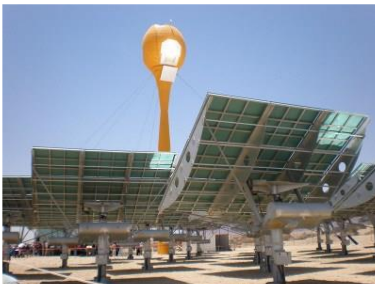
Figure 68. General view of the AORA solar tower facility.
