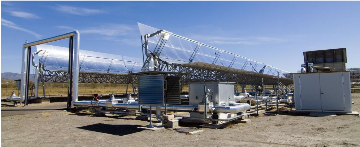
Figure 57. View of the IFL experimental facility (with parabolic troughs) using compressed gas as heat transfer fluid.
