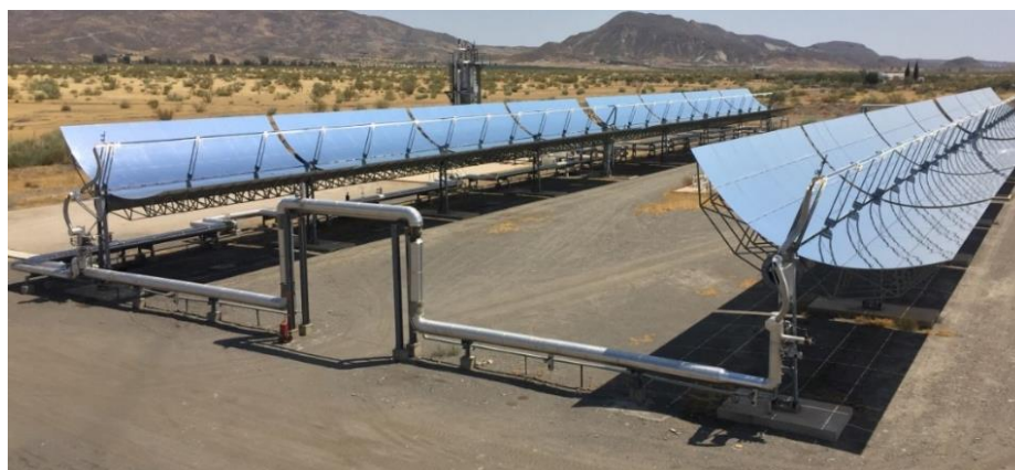
Figure 15. PROMETEO test facility used at PSA for HELISOL®XLP proof of concept.
