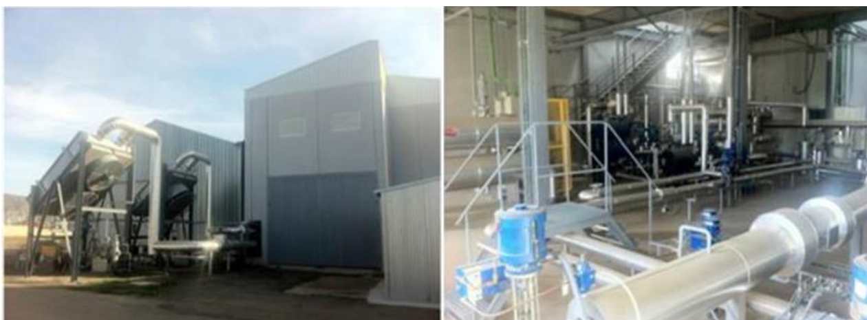
Figure 89. View of the outside of the CSP+D test bed building with the air coolers (left) and partial view of the interior of the CSP+D test bench (right).
