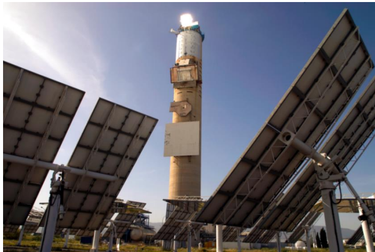
Figure 64. The CESA-I facility seen from the north.
