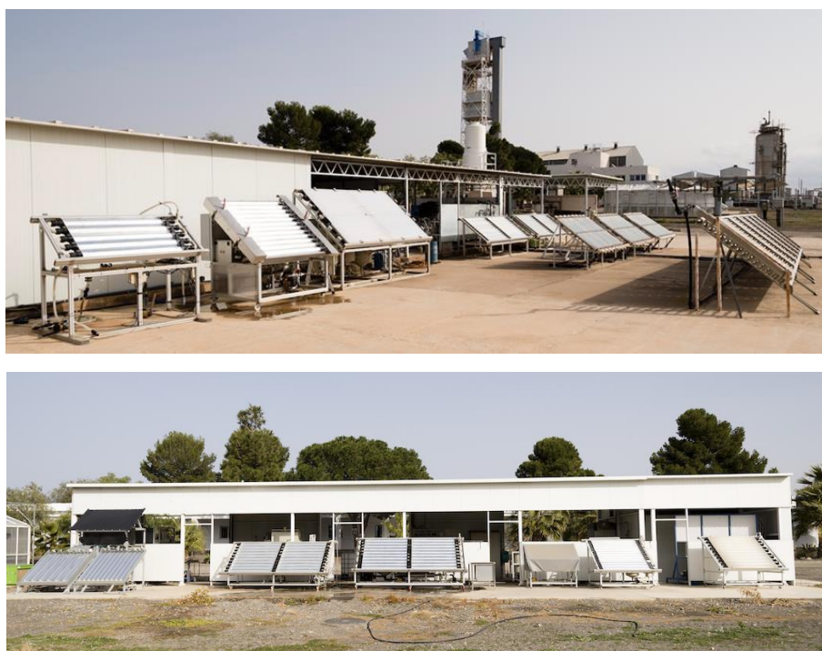
Figure 91. View of several CPC photo-reactors for purification of water. (top) CPC facilities I, (bottom) CPC facilities II.
